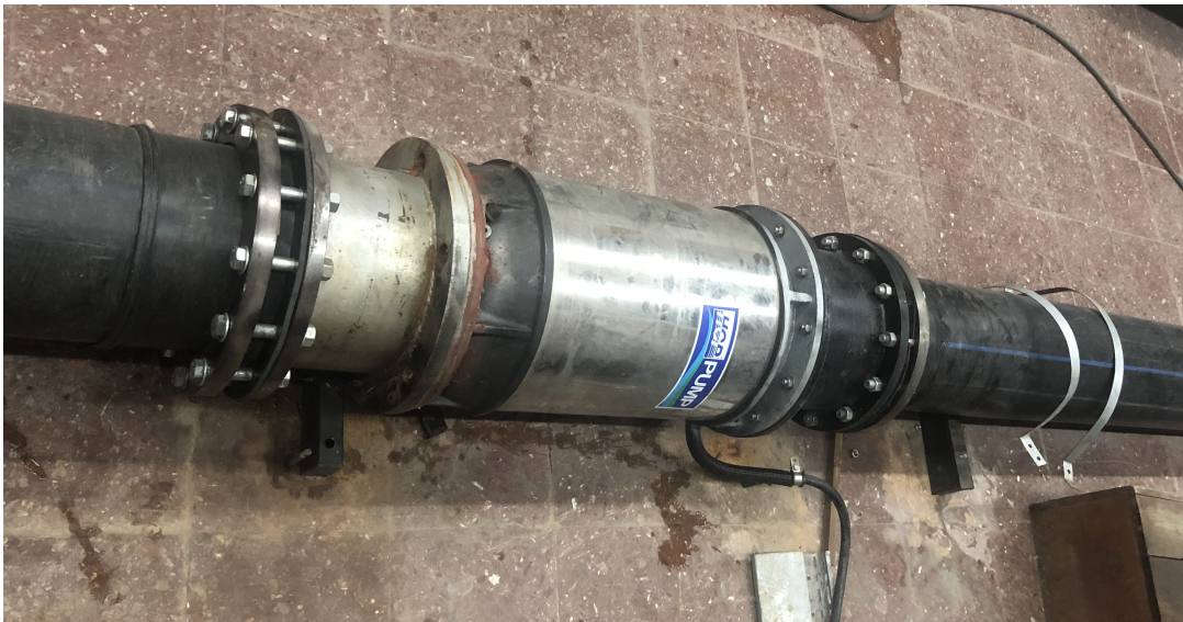
Figure 2.2: A photograph of one of the HPC L-300A Pumps
